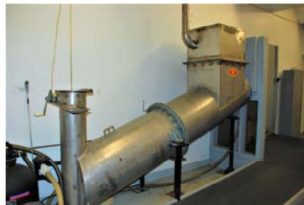
Figure 2. Horizontal water recovery tank
